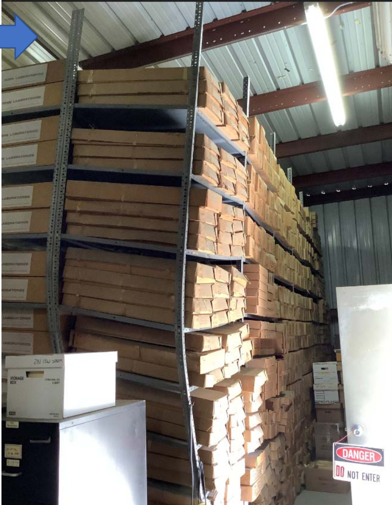
Earthquake bracing is not secured
